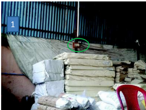
Electrical connections without industrial plug.
