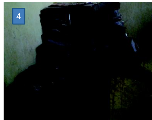
Combustible material stored in staircase.
