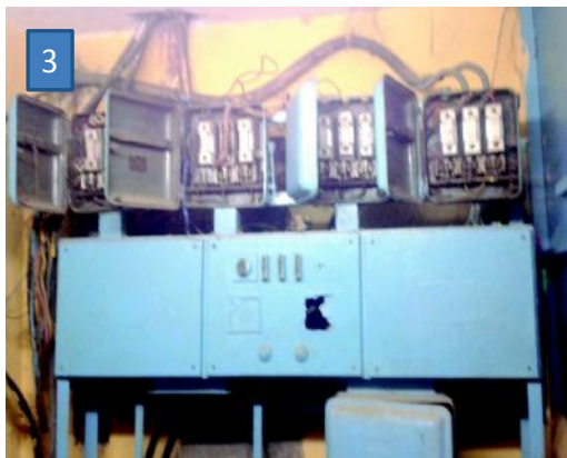
Unsafe electrical connections.
