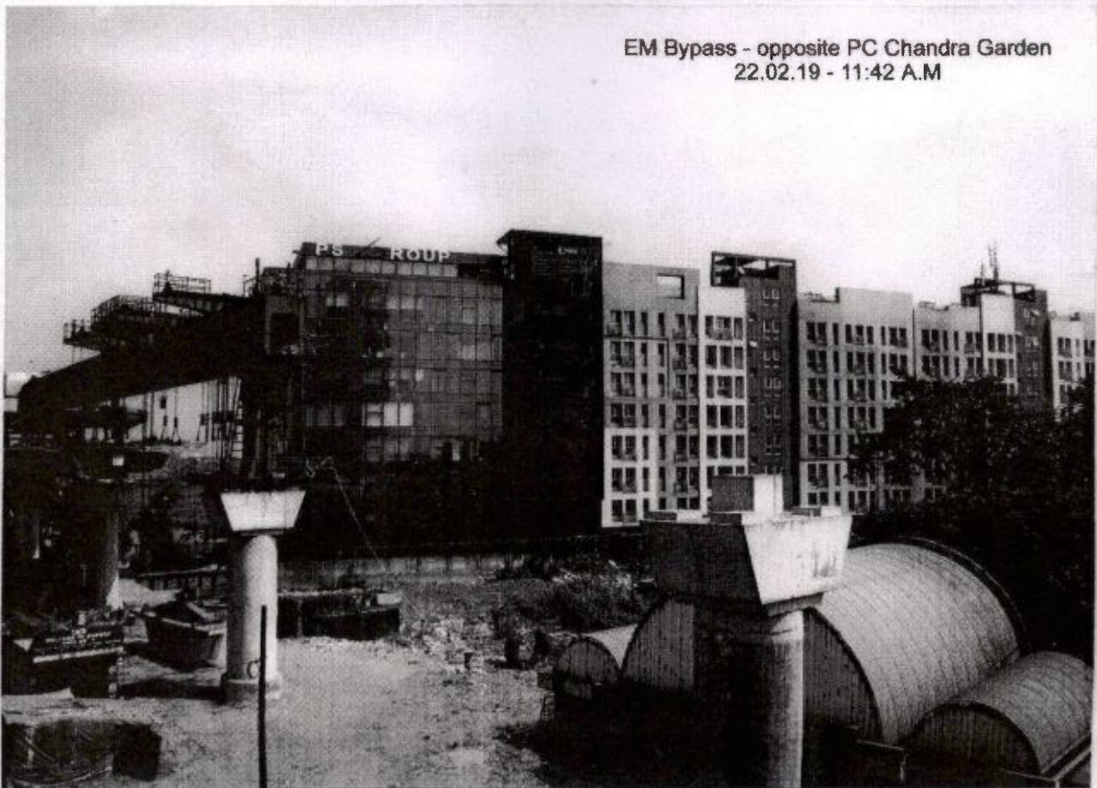
Photographs taken on 22.02.2019 showing Construction of Buildings opposite to P. C. Chandra Garden
