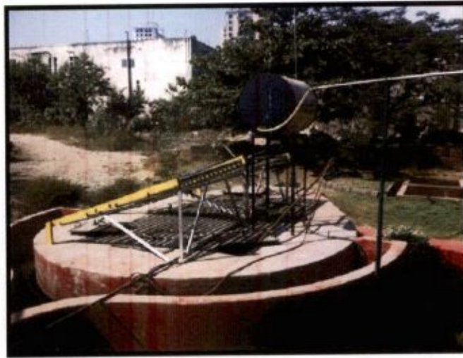
A Typical Pre-Digester
