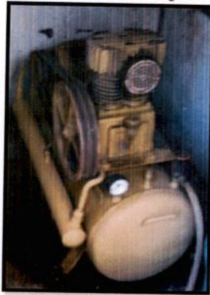
Typical Air Compressor
