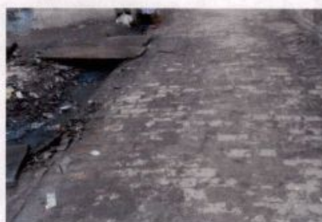
Image: Chocked Condition of Kuccha drain in Uttar Badra Slum
