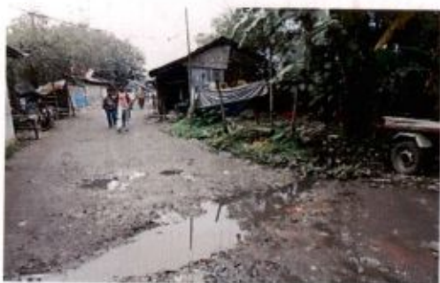
Image: Dilapidated condition of road at Bukra Slum
