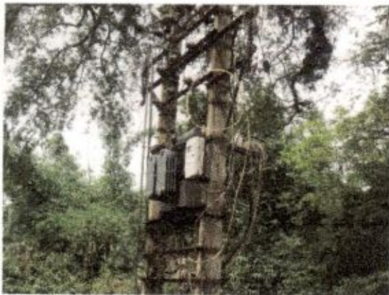
Transformer at ward 20
