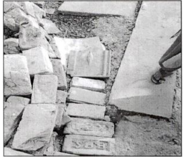
Fig.5. Blocked drain covered with tiles;
